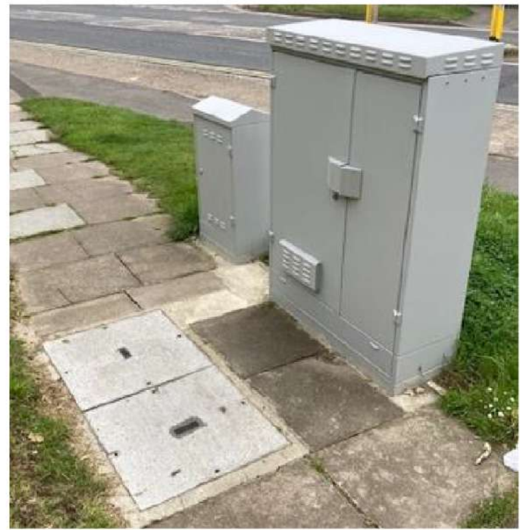
Example POP-A with SD1 Power Cabinet
